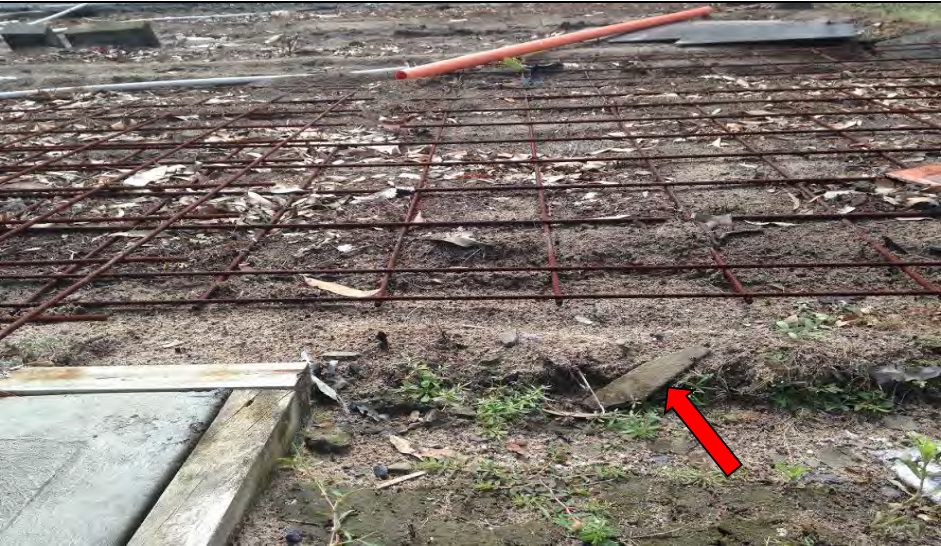
Photo 1: Suspected asbestos containing fibre cement fragment near gas storage facility in Norville Depot.
