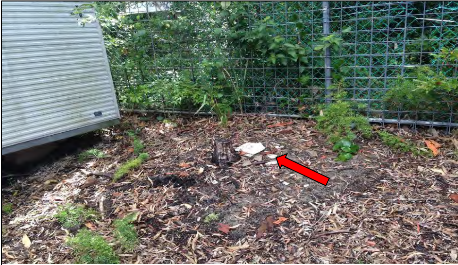
Photo 3: Asbestos fibre cement fragments near northeast corner of Building 2.
