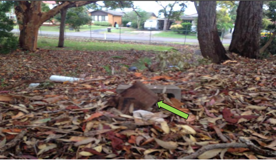
Photo 3: Non asbestos containing fibre cement fragment on south side of Building 6 near awning.
